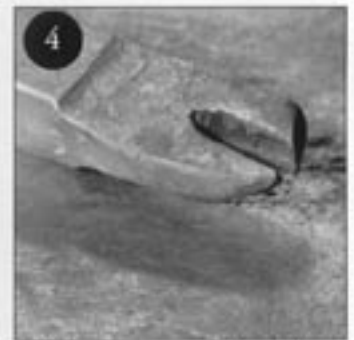
Hot cut on centerline 3/4" long
