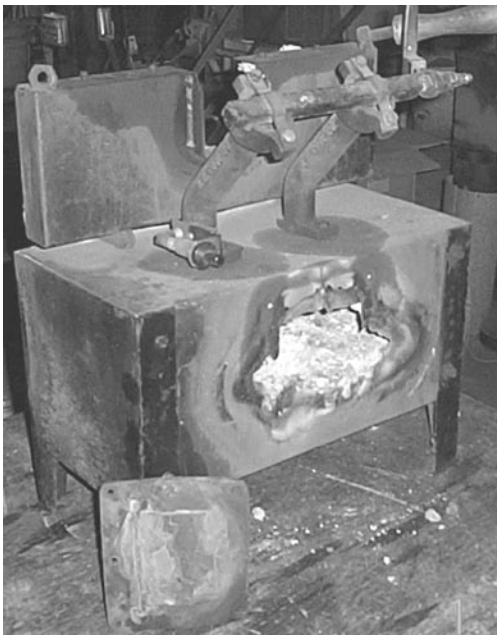
Left, Back wall of forge before repair.
