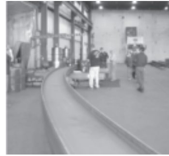
Cover Photo, Bending an I beam the hard way. More pictures on page 8.
