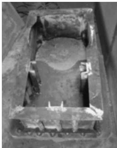
Base construction, web stiffening angle iron welded to I beam with three channel irons for extra support. I cut the flange of the I beam to make room for the flange on the anvil.
